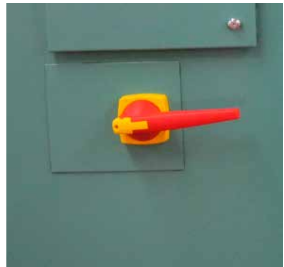
FIGURE 1 - EMERGENCY SHUTDOWN HANDLE
